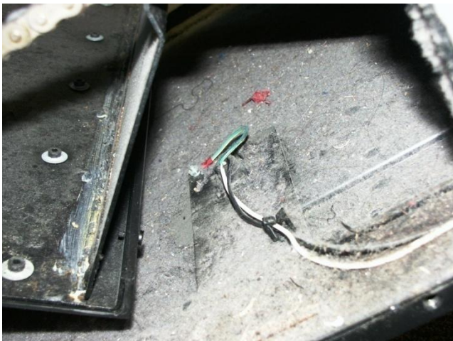
Figure 2. Input Power Wires
