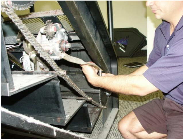
Figure 1. Loosening Bracket at the Frame End
